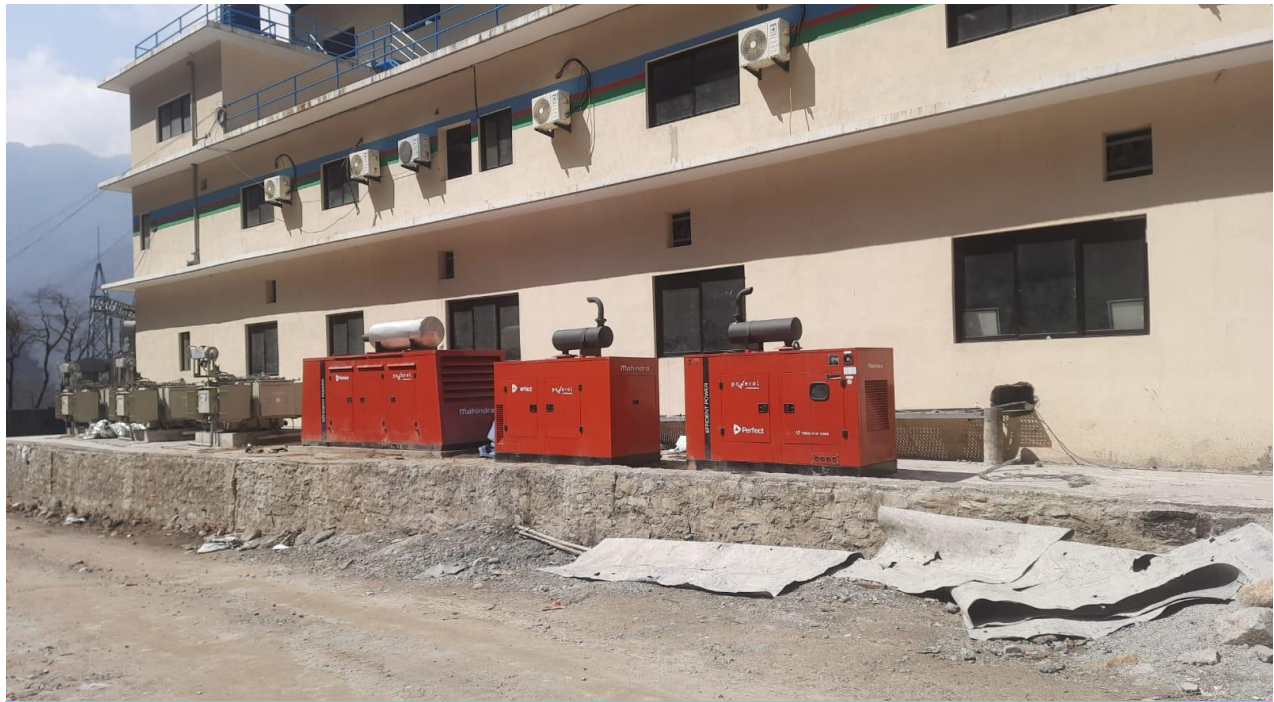
Backup Generators of PH and Both Headworks
