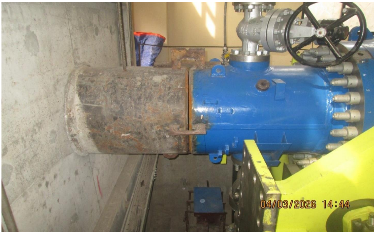
MIV alignment with Turbine Bifurcation
