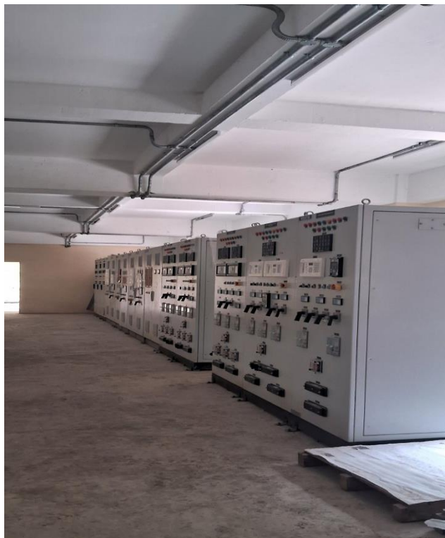
Control Panel in Control Room
