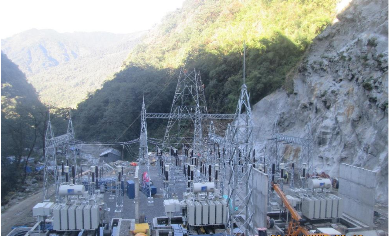
Sending End Switchyard
