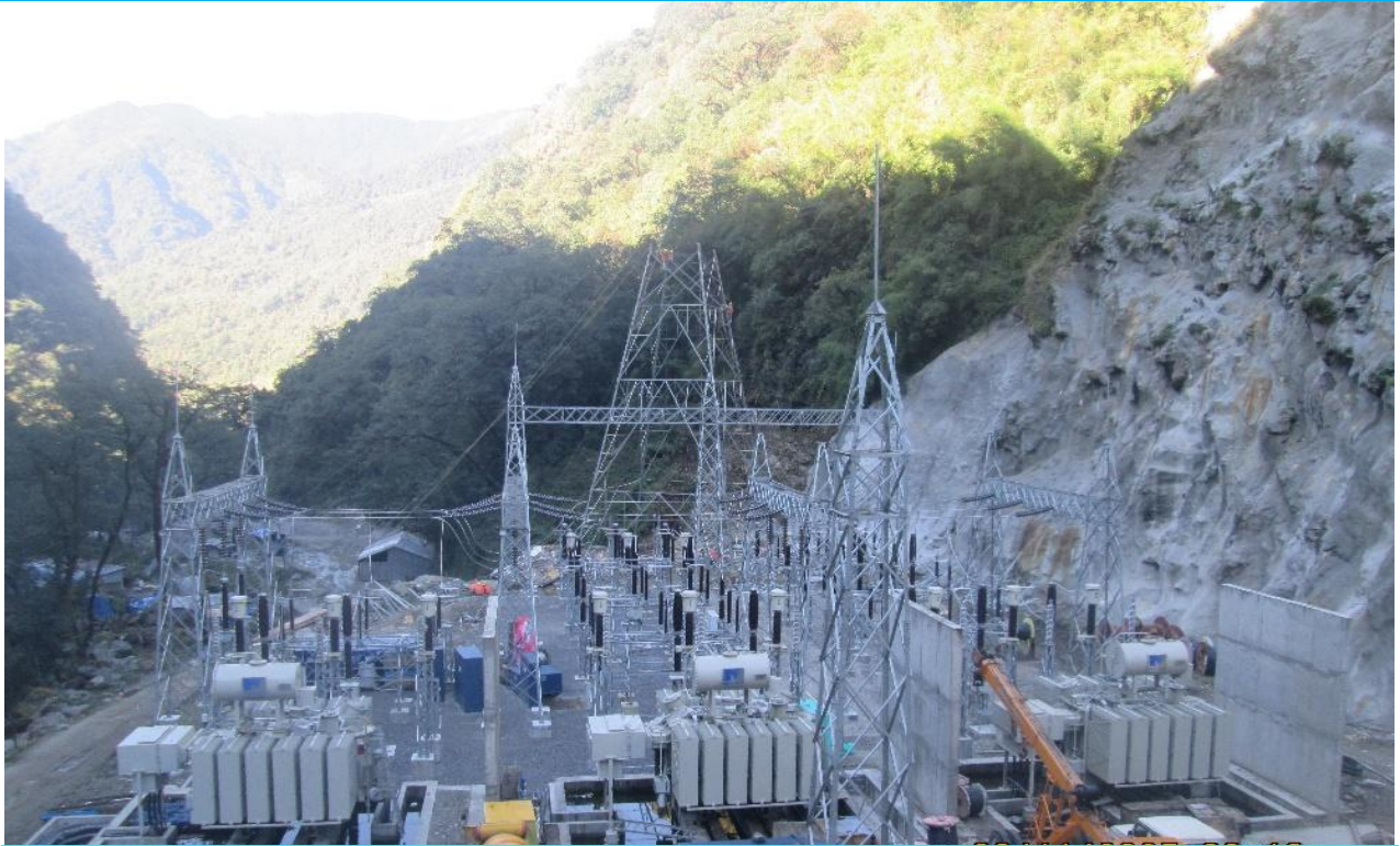
Sending End Switchyard
