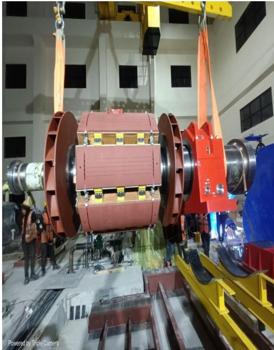
Assembled Stator and Rotor of Generator
