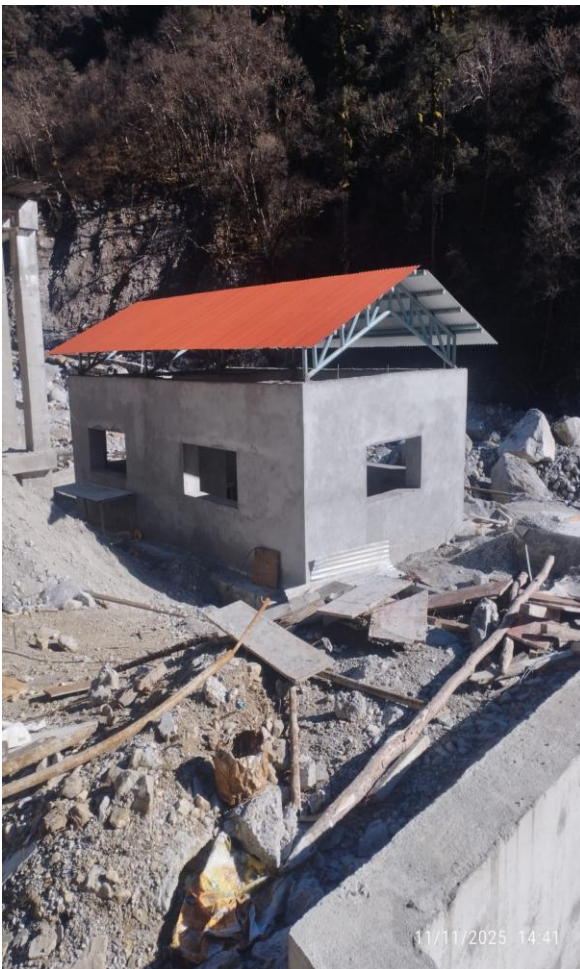
Control Room at Likhu H/W
